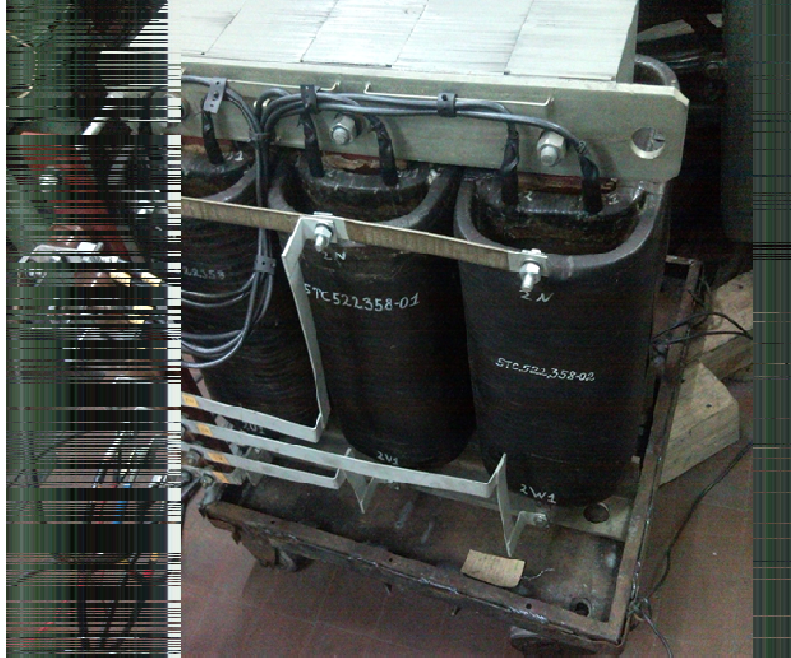
Figure 2. Three-phase transformer T-164 with the scheme and winding connection group Dyn7 for usage onboard of electric locomotive
